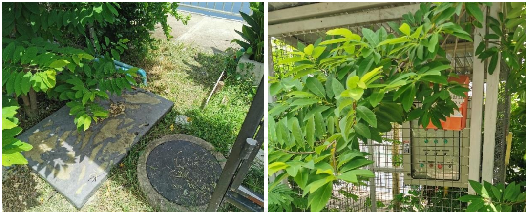
Figure 4.8 Waste Water Treatment System of the Community.
