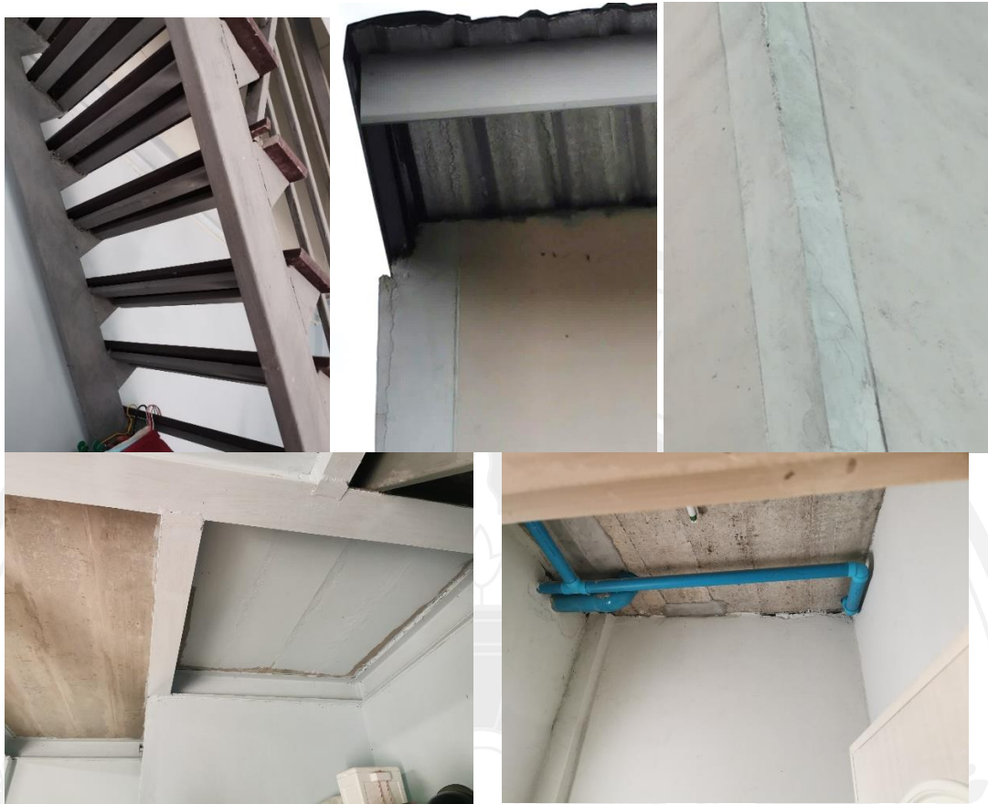
Figure 4.18 Quality construction problems.
